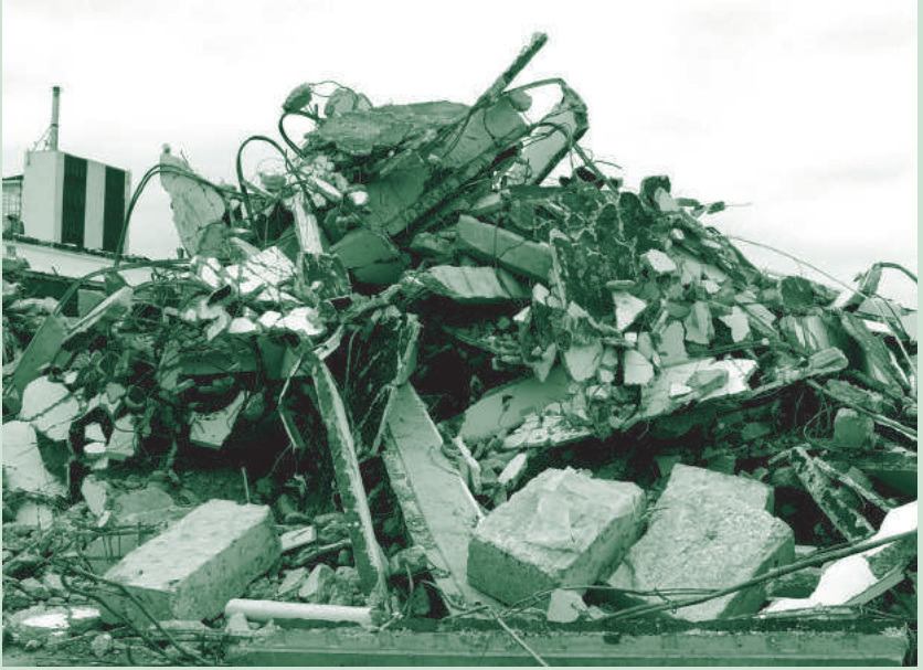
Photo: Demolition site with piles of downcycled materials with low or no value as resources for future buildings.
